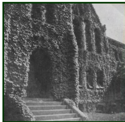
Ivy, taken from John Wesley's grave, that once covered the church was removed because of structural damage. The picture was taken about 1907
